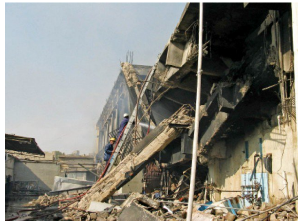
Figure 7 Goods worth millions of rupees were completely destroyed, while part of the building collapsed (Source: The Express Tribune).
