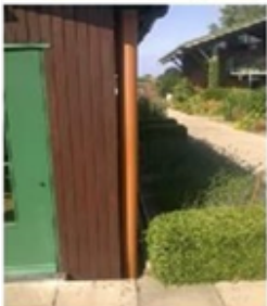
Figure 6 During summer months, the tap is left open to supply the plants with maximum rain water after a light down pour, and during heavy rainfall, the pipe is flushed through to remove sediments.
